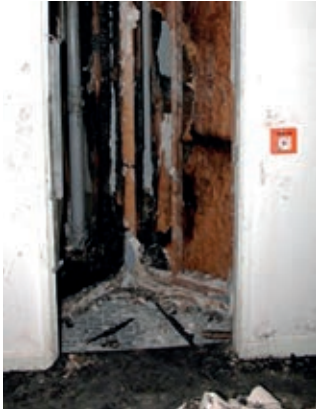
Example of fire spread within voids of a timber framed building, extending to floors beyond the initial fire origin.
