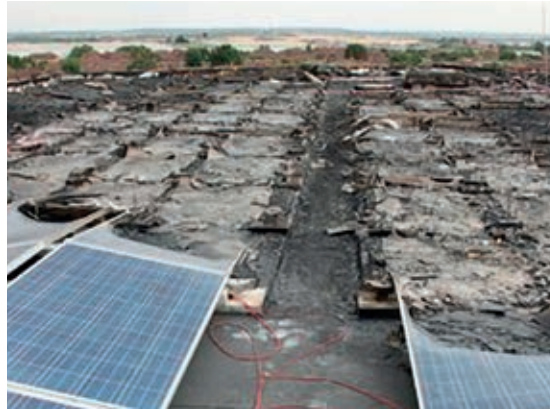
Extensive fire spread at PV panels on a new-build roof.
